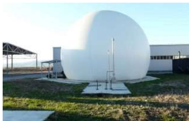
Wastewater Treatment Plant (WWTP) in Kočani, Macedonia.
