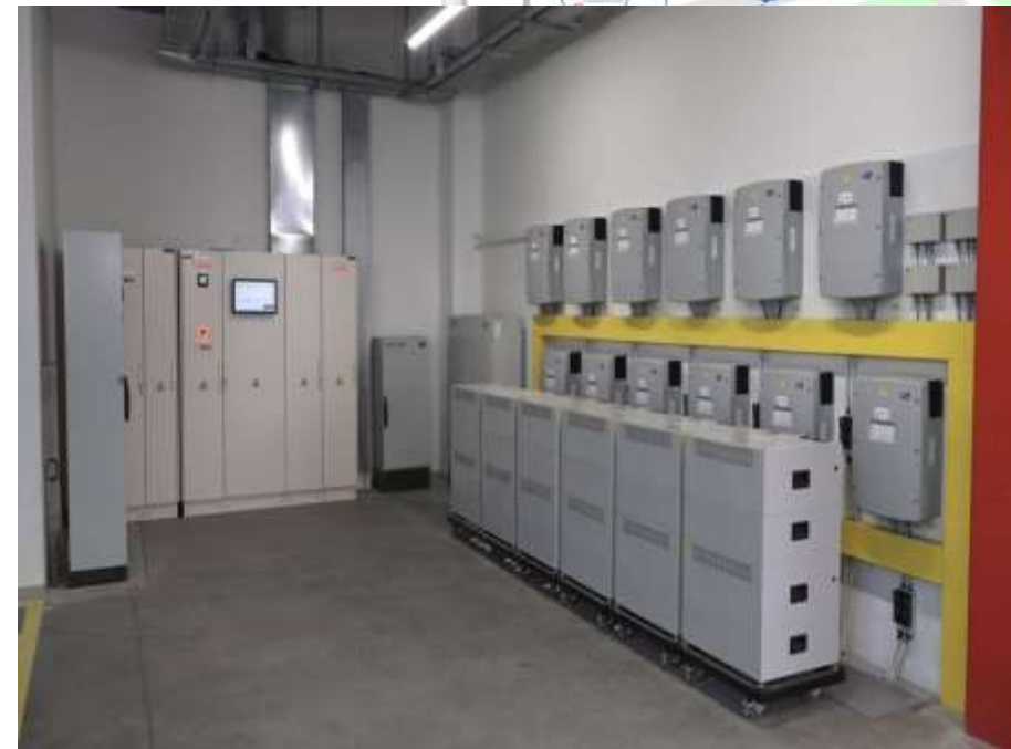
Photovoltaic system (panels, inverters, batteries) and power monitoring system
